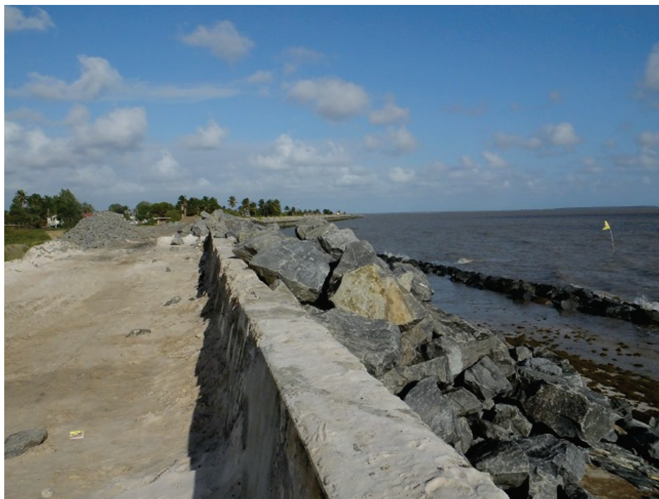
Sea Defense Work is taking place involving the placement of riprap in front of the seawall.
