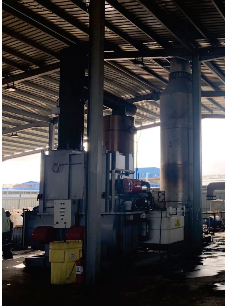
Figure 2.10-6: Vertical Infrared Unit with Wet Scrubber and Oxidizer at Typical Waste Management Facilities
