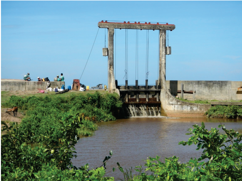
Figure 8.1-9: Sluice Gate (Koker) in Charity (Region 2) at High Tide
