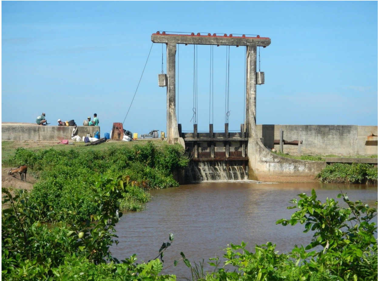
Figure 9.1-10: Sluice Gate (Koker) in Charity (Region 2) at High Tide
