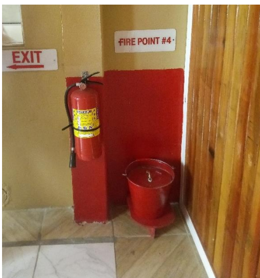
Figure 9: Fire extinguisher and sand bucket at one fire point
