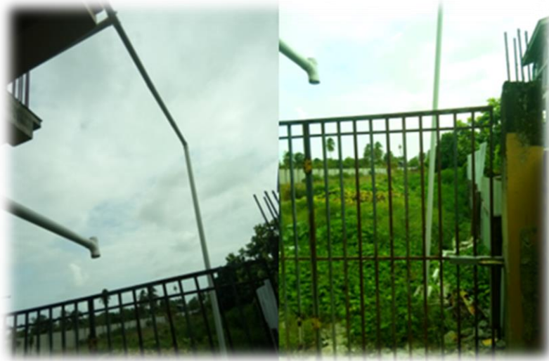
Figure 2: Pipes extending from hotel to drain in empty lot south of the hotel
