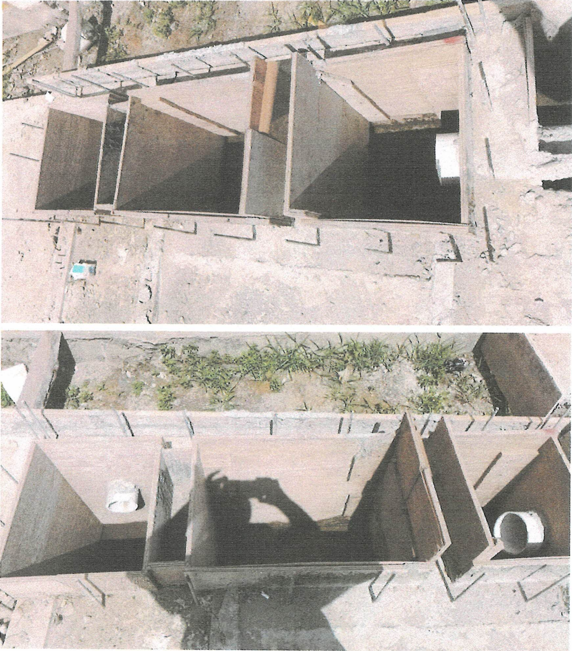
Figure 5. Pictures of oil water separator at the service station (construction to be completed)
