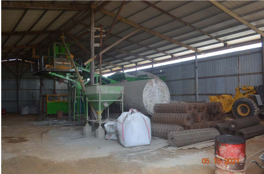
Photo 7: Existing Mini Concrete Plant
