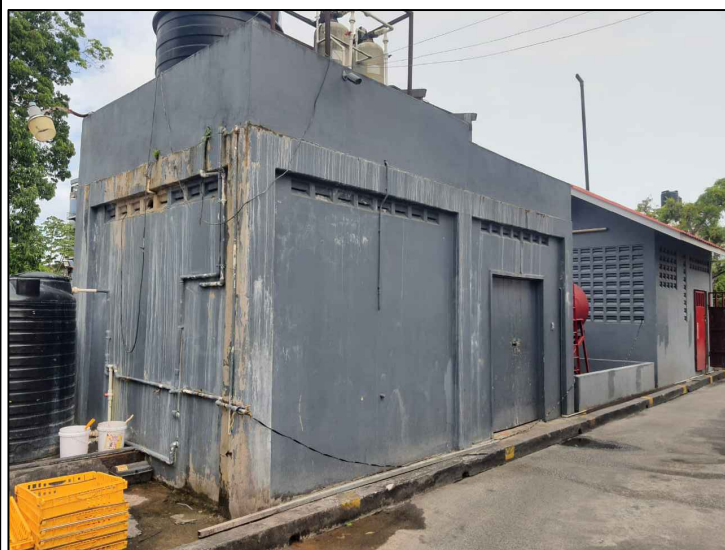
Water Supply & Filtration System
