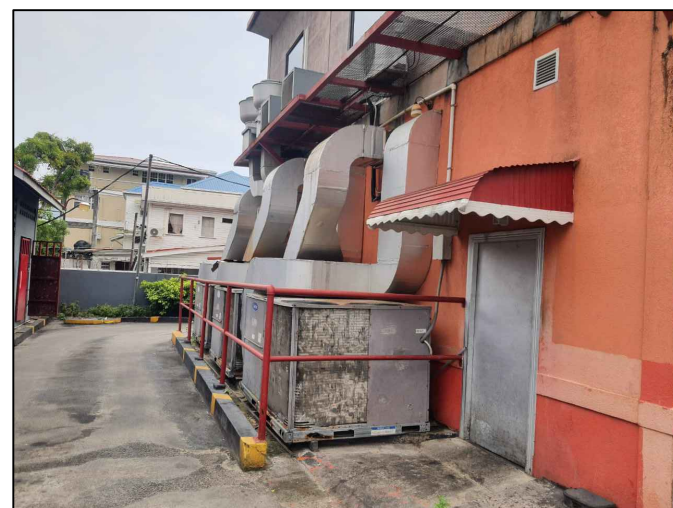
Central Air Conditioning Unit
