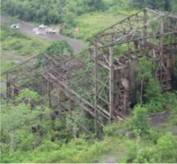
Figure 17-3: Skeleton of Former Processing Plant at Matthew's Ridge
