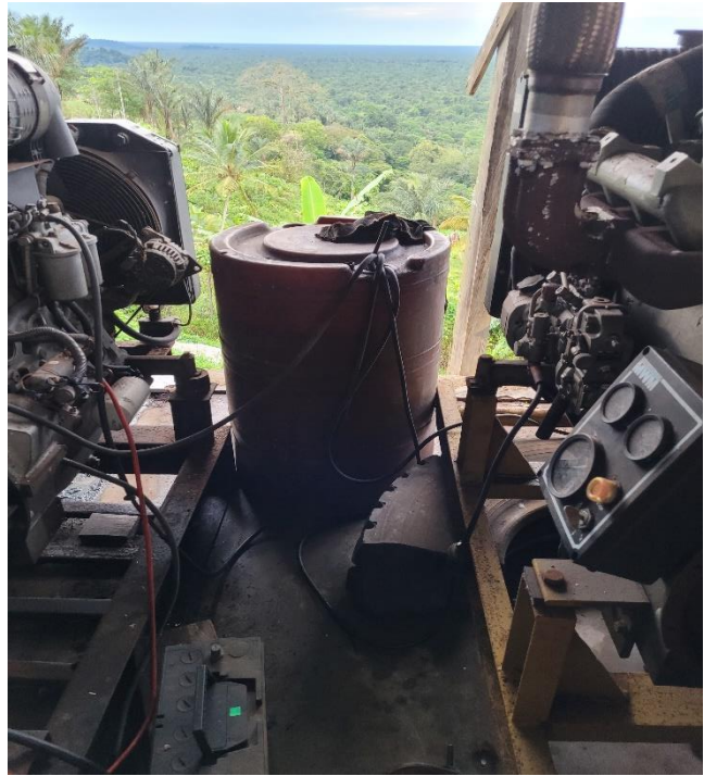
Showing the smaller container for the generator
