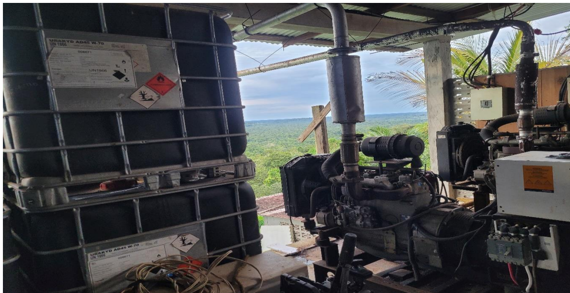
The storage tank with the generator
