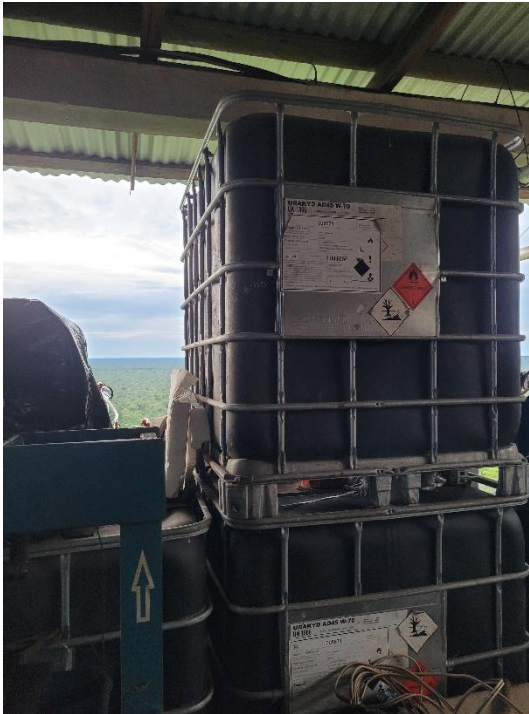
Inside view of the storage tanks (totes)
