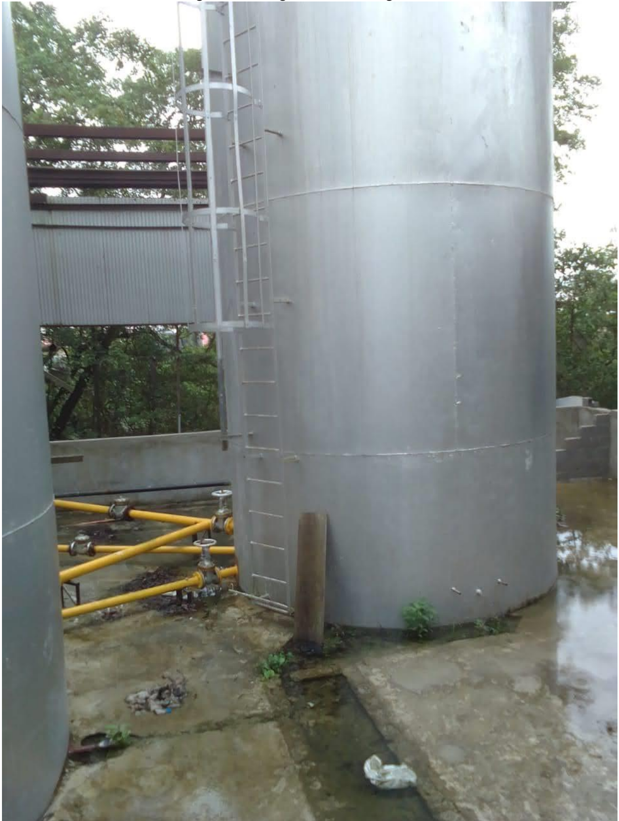
<Figure 9: Aboveground Fuel Storage Tank>
