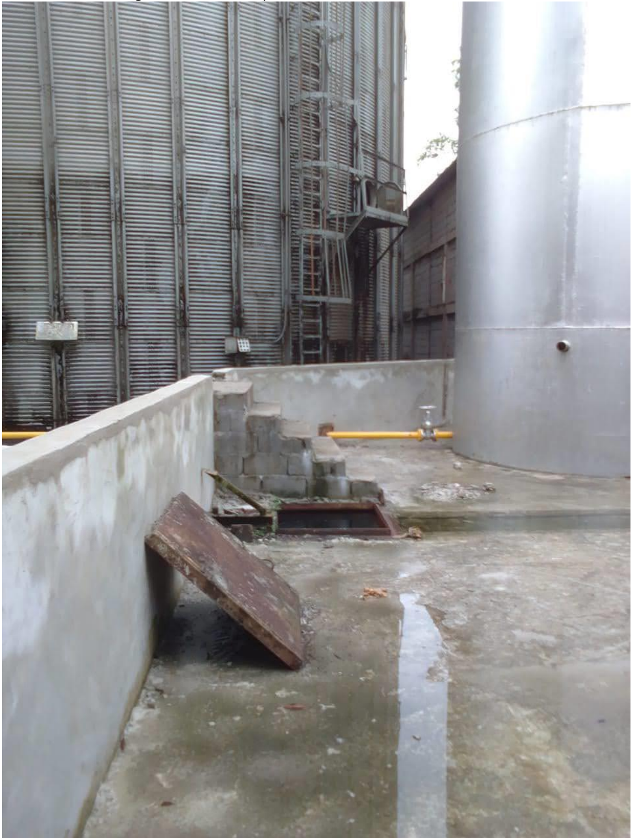
<Figure 10: Oil Water Separator inside of Fuel Containment Bund>
