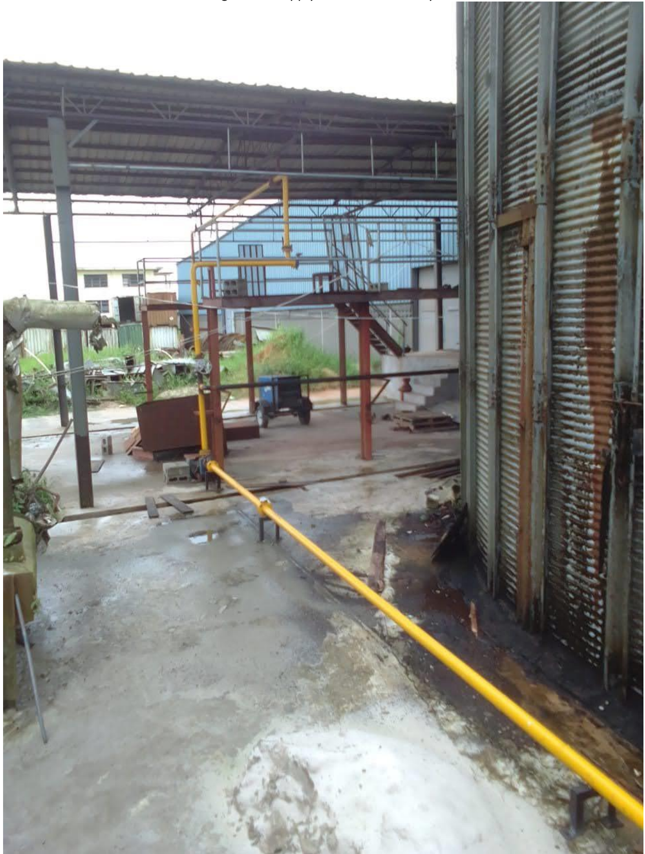
<Figure 11: Supply Line to Fuel Gantry>
