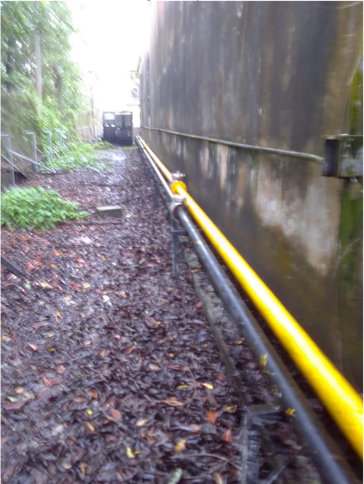
<Figure 7: Fuel Pipelines>
