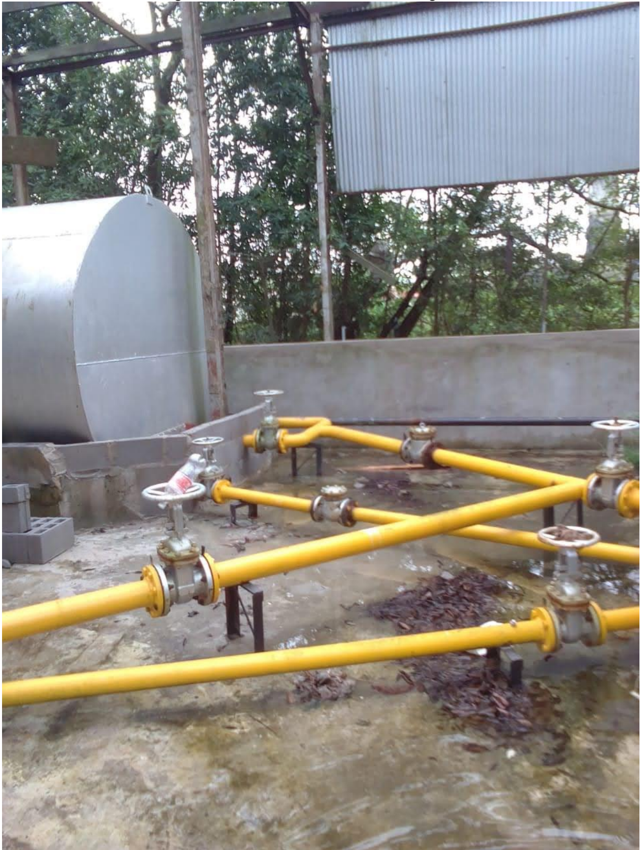
<Figure 8: Pipelines with Valves to Fuel Storage Tank>
