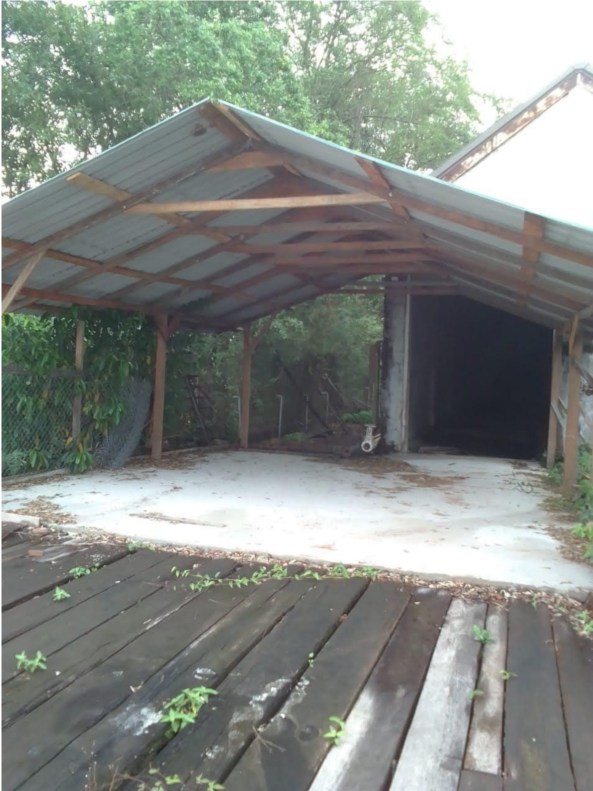
<Figure 6: Fuel Intake/ Outlet Point>
