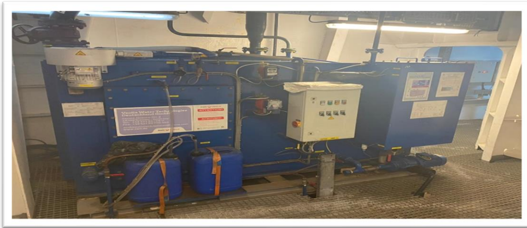
Image 15: Sewage Treatment Unit
